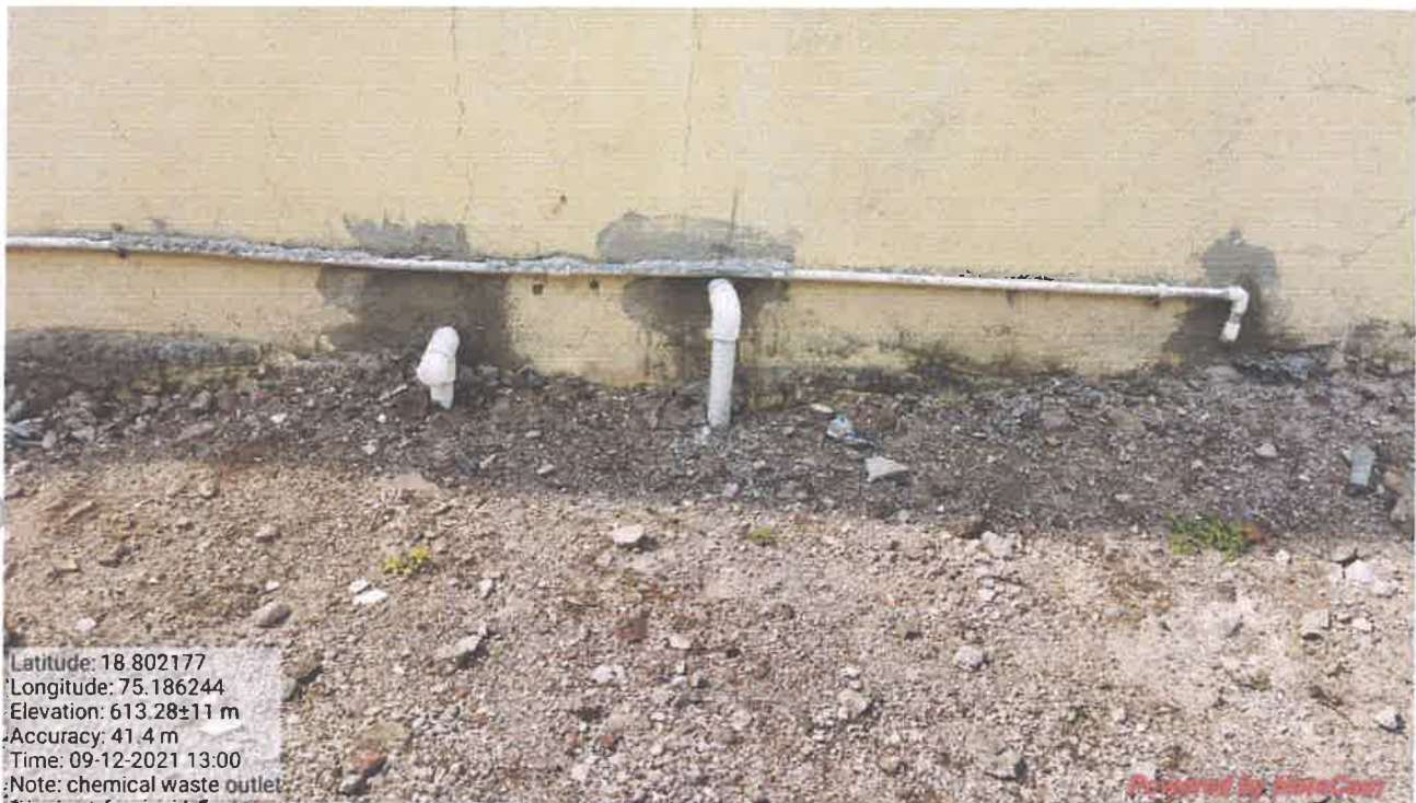
Hazardous Chemical Waste Outlet
